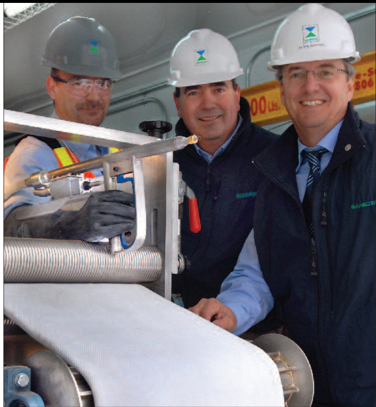
Sanexen Environmental developed Aqua-Pipe in 1999, addressing the lining of water drinking water mains. From left are Pierre Jomphe, Aqua-Pipe foreman; Ben Côté, Aqua-Pipe vice president; and Alain Sauriol, Sanexen Environmental Services president.
